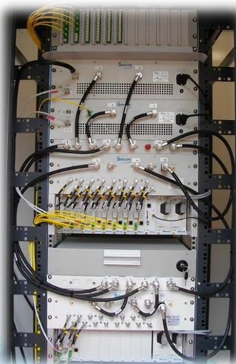
Wiring on a rack with 10 fiber optic distribution
